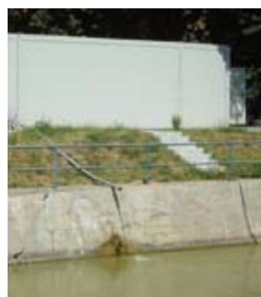
View of the container from the river side including pumping and outlet facilities.
